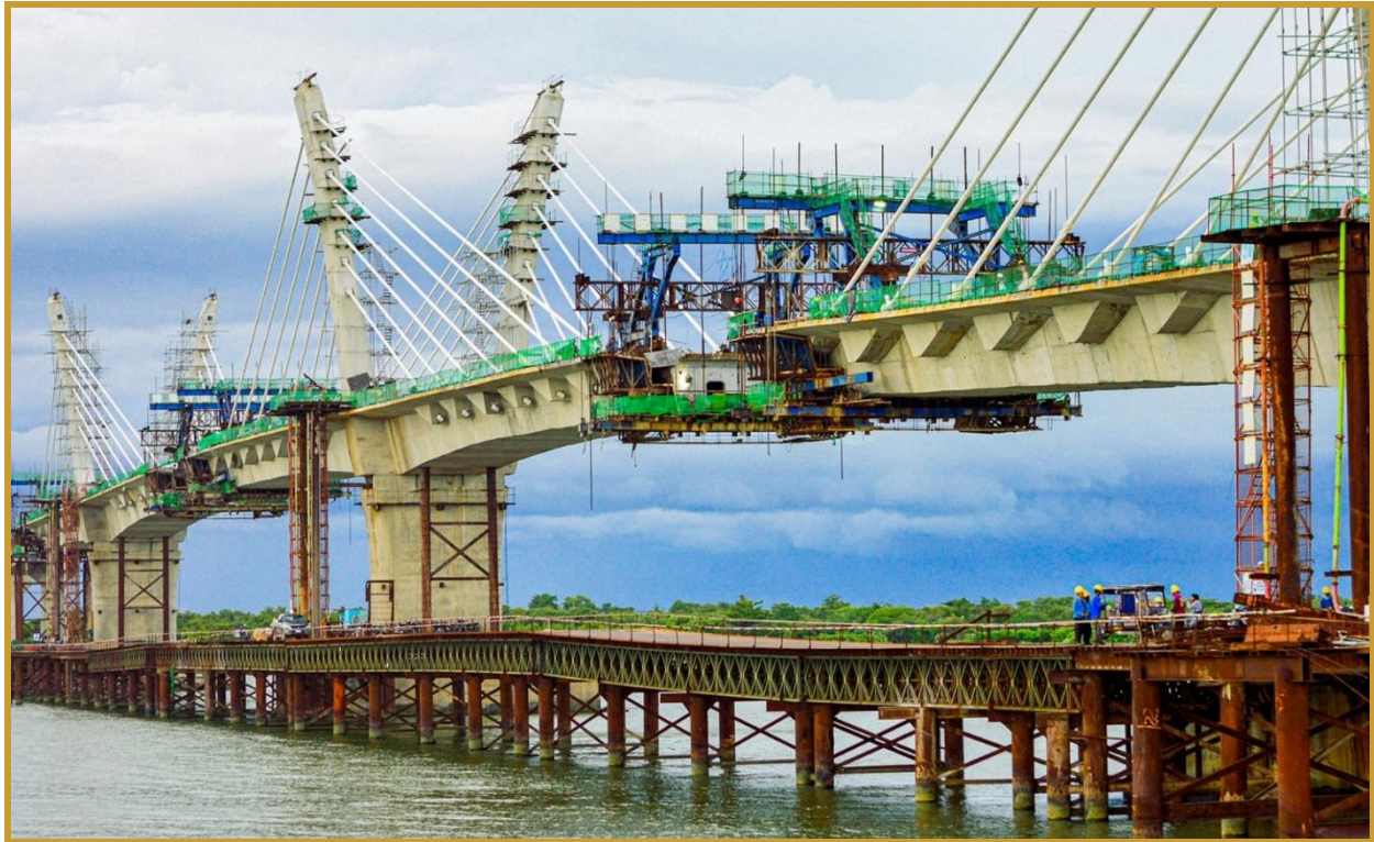
Construction of the Camalaniugan Bridge connecting the municipalities of Aparri West and Camalaniugan.
